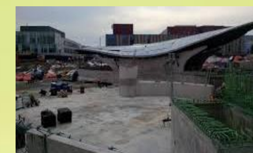
York University Subway Station, planned for the Pan Am/Parapan Am Games Toronto
